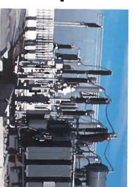
Power Plant Substation
