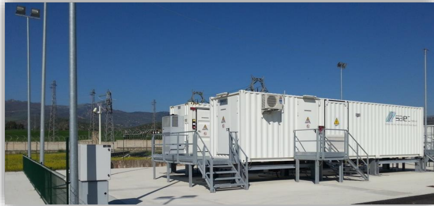
ENERGY STORAGE \leq 1 MW
